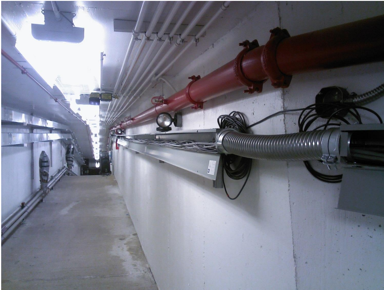
Figure 1 HD Tagger Ramp PSS Installation
